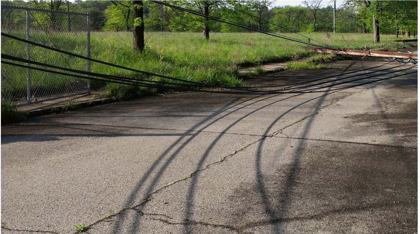
Fallen over electric poles at the gate to Bonifay St.
